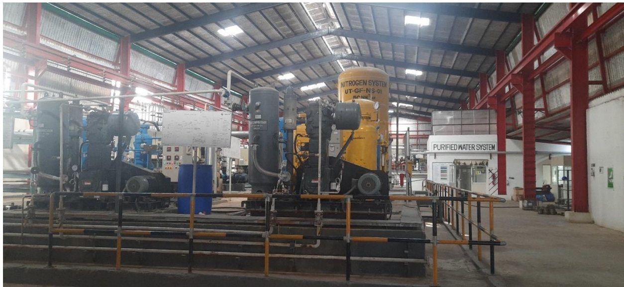
Inbuilt Water system facility at Almelo Pharmaceuticals
