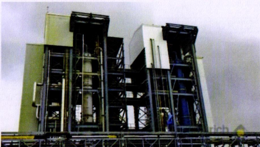
Bromine Production Plant
